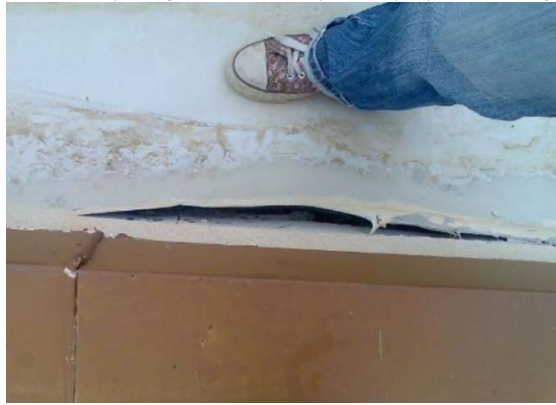
Figure 2. Deficient tail-end between the waterproofing membrane and the perimeter parapet. Source: image by Manuel J. Carretero-Ayuso.
